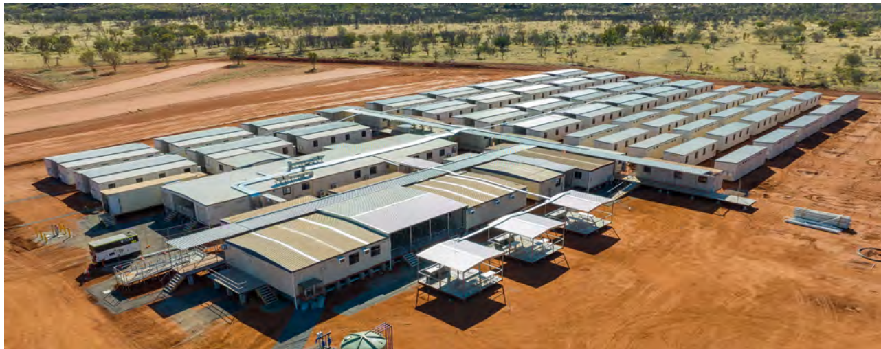
Figure 3. An aerial view of stages 1 and 2 of the construction camp, with capacity to accommodate up to 200 people.
